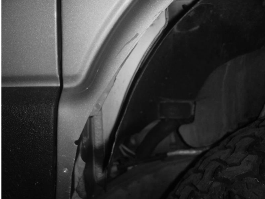
The Passenger Fender at the cab after being cut. Note the small 5/32" hole about 1/2" from the door gap.
