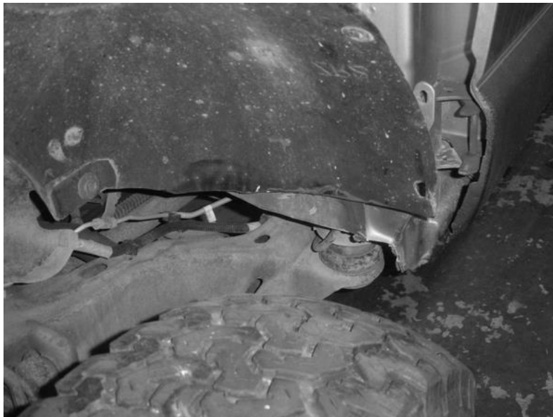
The fender liner after being cut. You will need to push the liner closer to the cab to stay inside the new flare. (Driver's Side)
